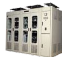
Subway Substations (Silicon Rectifiers)
