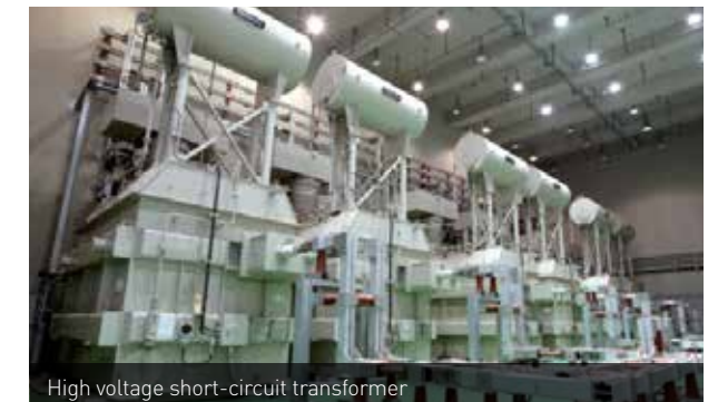
High voltage short-circuit transformer
