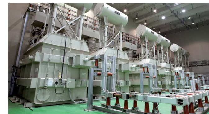
High voltage short-circuit transformer
