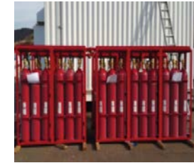
Fire Fighting System
