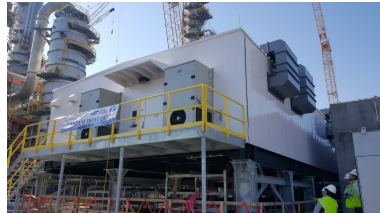
E-House (Prefabricated type)
